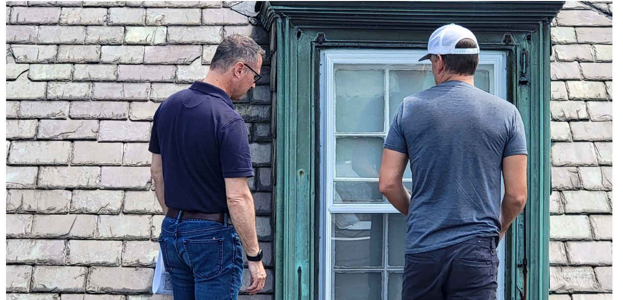
Tom Connolly, AIA of Connolly & Hickey, our historic preservation architect, with Glenn Crooker, Jr. of Alden Bailey, the contractor who executed Phase One.
